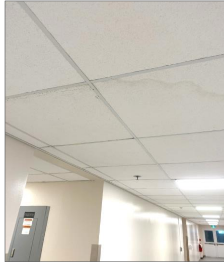
Photo 12 – Water-stained ceiling tile in Hallway.
