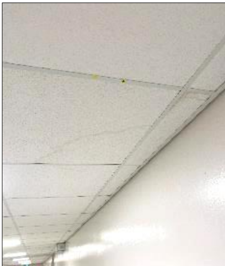
Photo 13 – Water-stained ceiling tiles in the Hallway.
