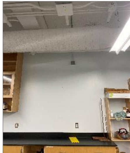
Photo 10 – West wall with elevated moisture readings approximately at six feet from ground, covering 9 ft 2 of drywall.
