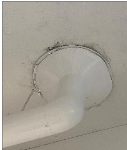
Photo to 8 –Cracks noted around ceiling vent.
