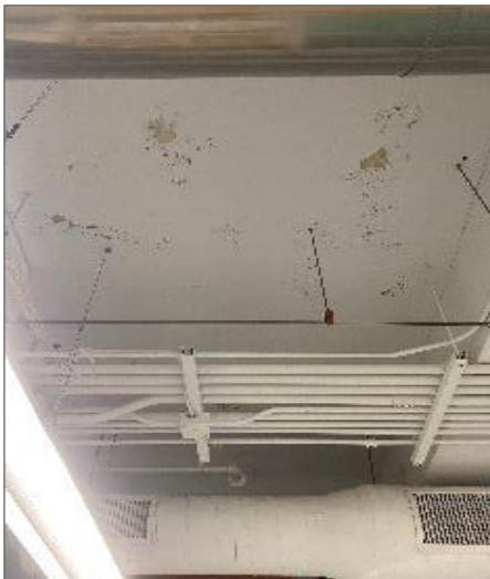
Photo 7 – Paint/Plaster peeling on the ceiling.
