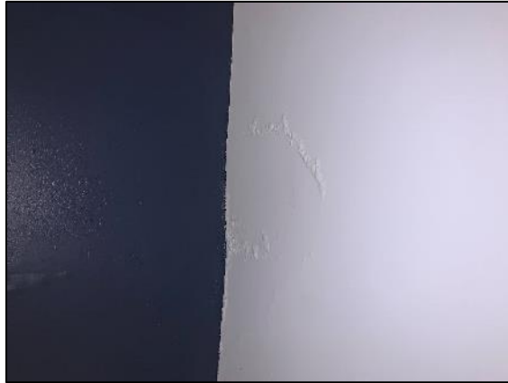
Photo 4 - View of bubbling paint and efflorescence on the south wall.
