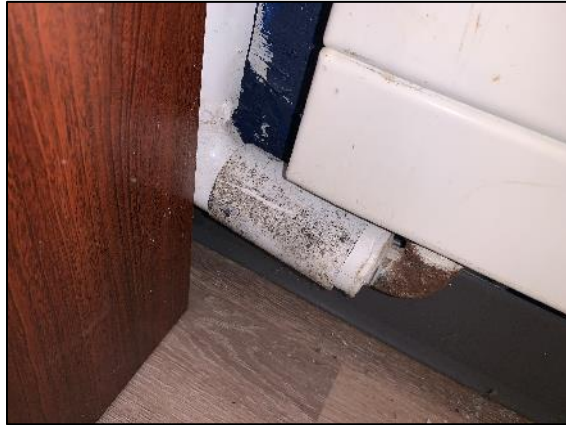
Photo 3 - View of mould growth on the pipe insulation.
